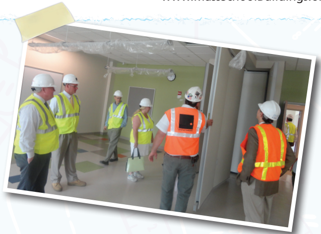
MSBA Executive Director Jack McCarthy and Project Manager Paul Fowkes, as well as Local Uxbridge officials, survey construction at Uxbridge High School.
