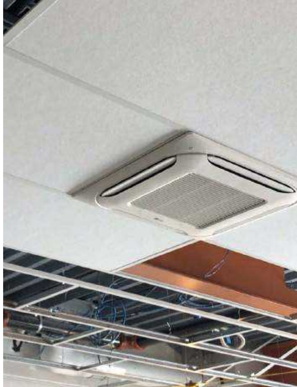
1 of 2 VRF ceiling cassettes installed in every typical classroom
