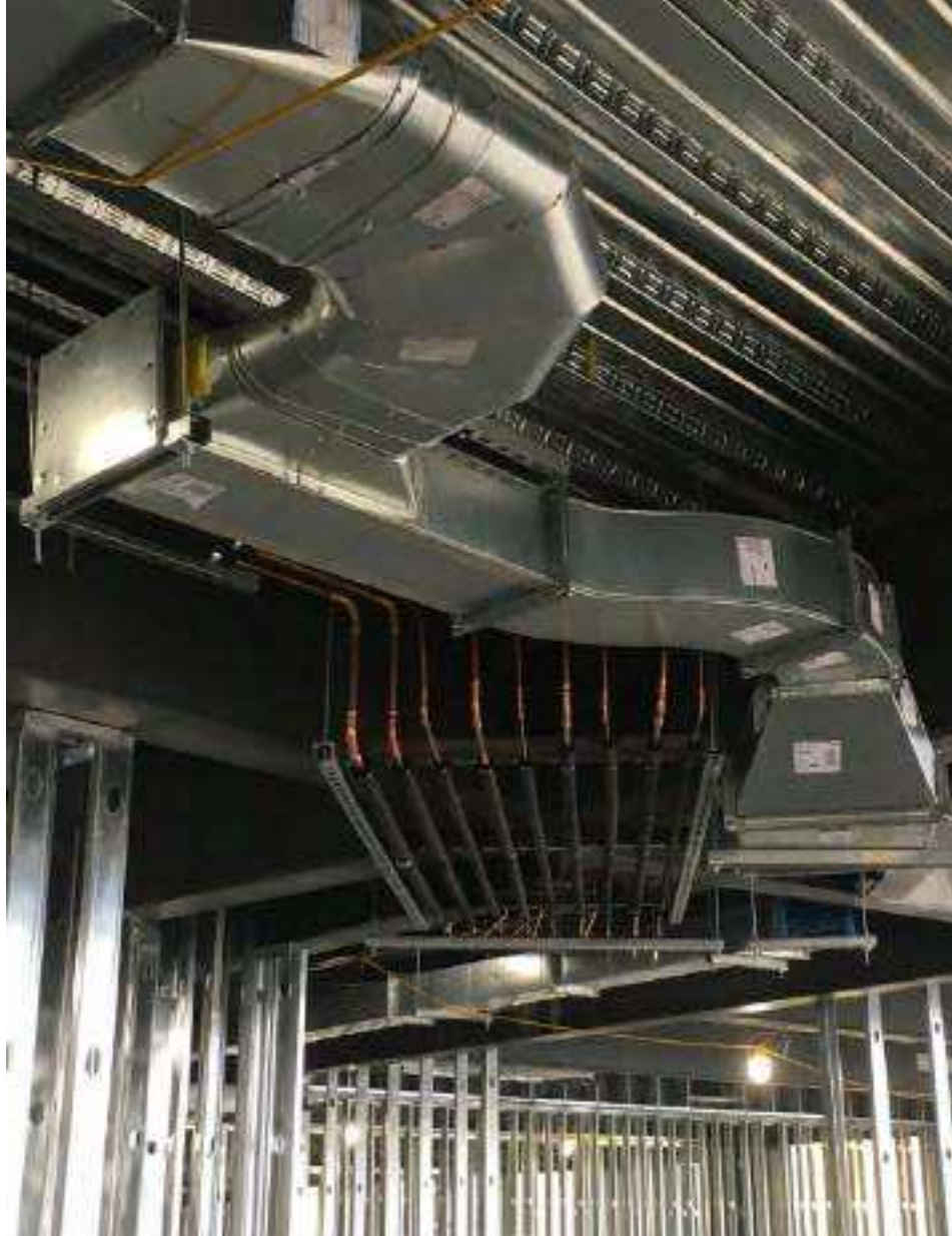
Ductwork and refrigerant lines were coordinated tight to steel
